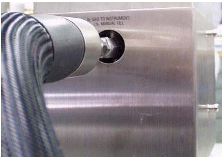
Figure 6 Coolant transfer hose attached to the GCA.
